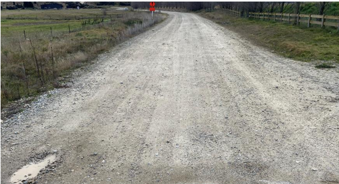
Figure 1.3 Corrugations on Queensberry Terrace.
