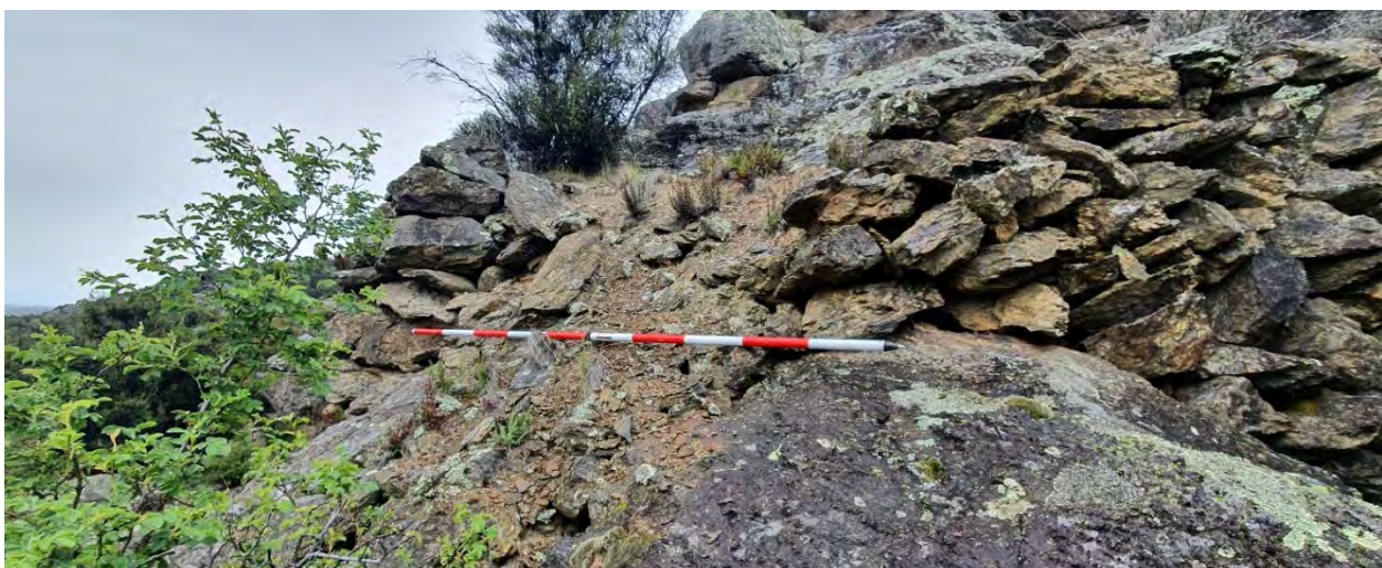
Figure 17. Partial collapse at NZTM E1308004 N5017209.
