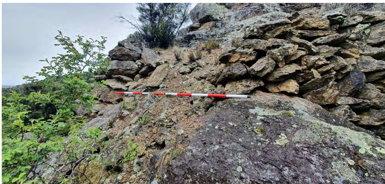
Figure 6. Partial collapse at NZTM E1308004 N5017209.
