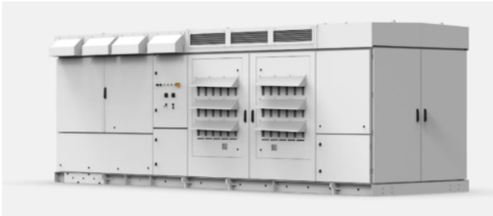
Figure 5: A typical Inverter
