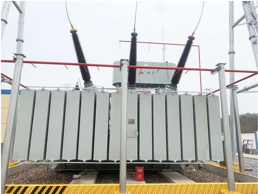
Image 3: 150MVA 33/220KV transformer
