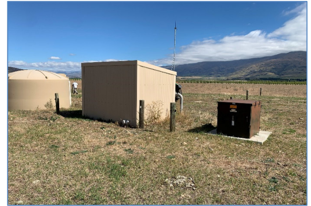
Photo 9: Well area with storage tanks, pump shed and electrical transformer.
