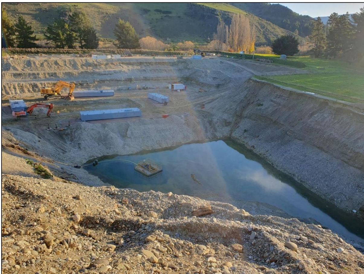
Figure 3: Works already undertaken on the site. Source: Council compliance site visit photos taken on 15 May 2023.
