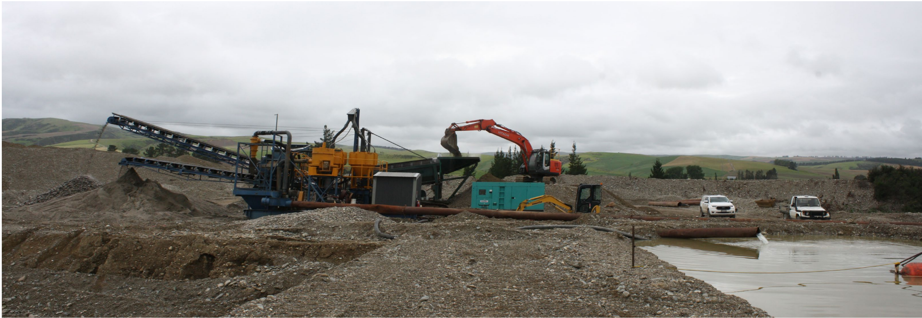
Figure 13: The processing plant already present on the site for the exploratory works.
