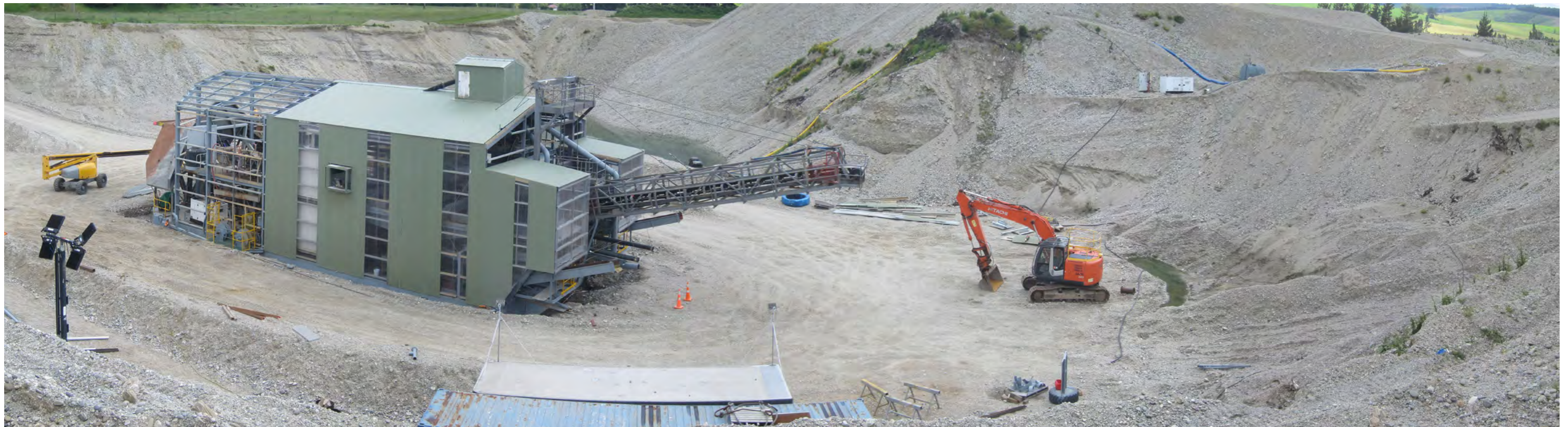
Viewpoint 4 - View of the dredge from within the site, the test pit and stockpiles can be seen behind the dredge.
