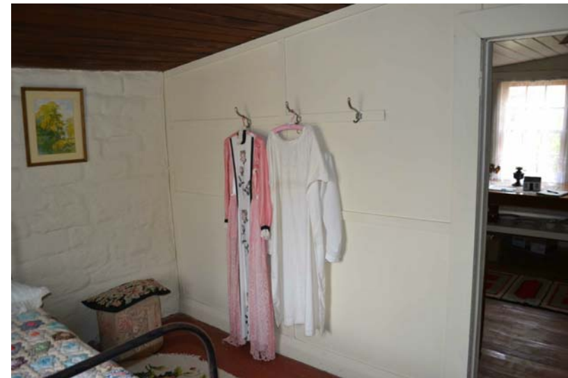
3. Room 3 showing the junction between the painted mudbrick wall and the timber framed lined and paneled internal wall adjoining the kitchen.
