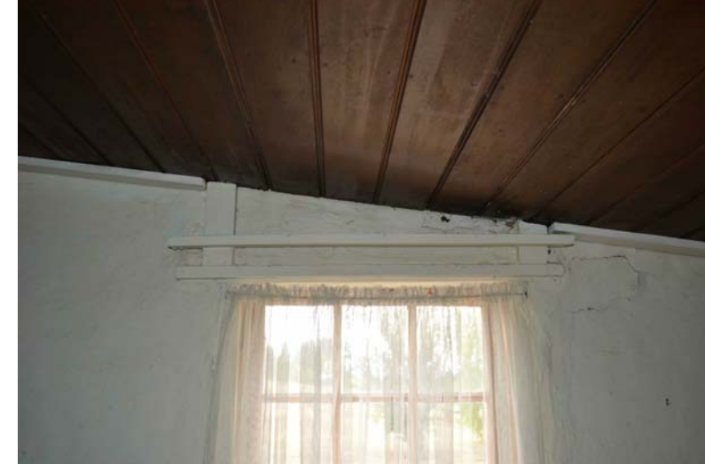
3. Room 3 Cracking to walls around window, missing architrave.
