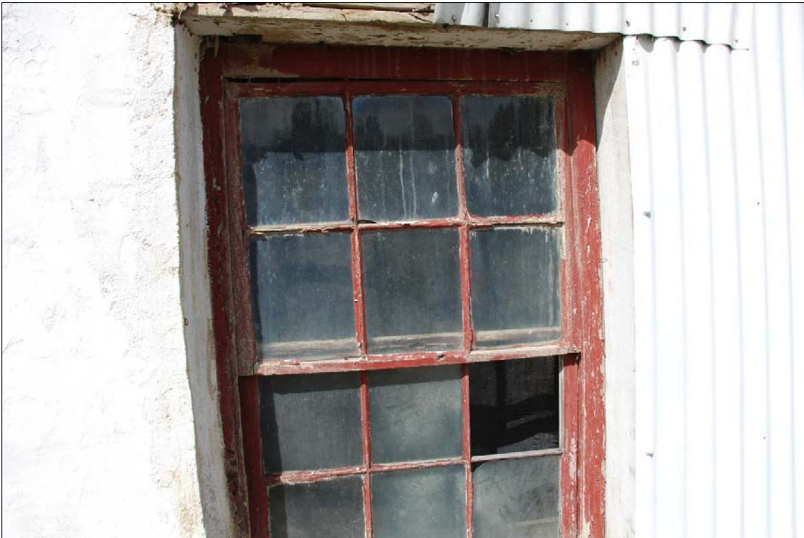
Figure 21: One of the six over six sliding sash windows at Peyton's Patch; it is almost identical to those at Vallance Cottage. Photograph: Origin Consultants
