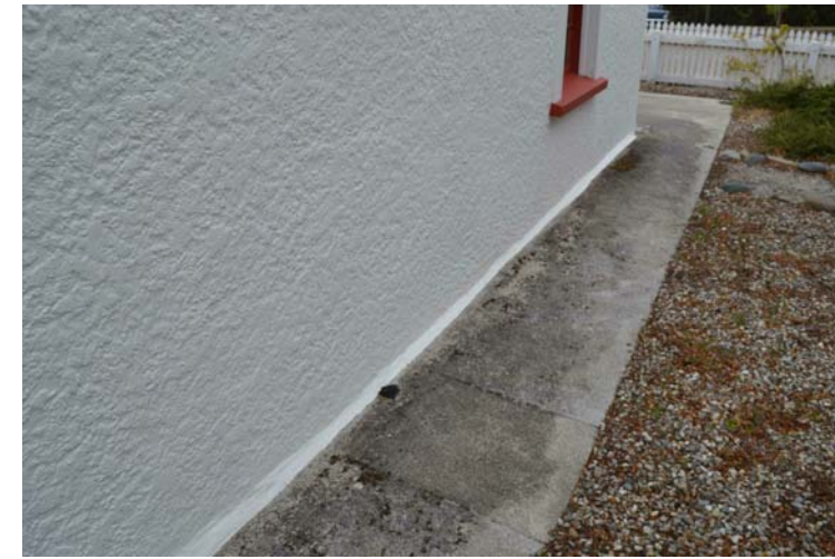
6. Plaster taken right down to ground/path level.
