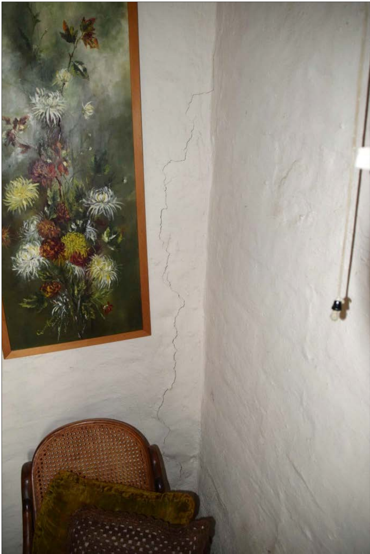
Figure 24: Cracking in the southwest corner of room 2. Photograph: Origin Consultants
