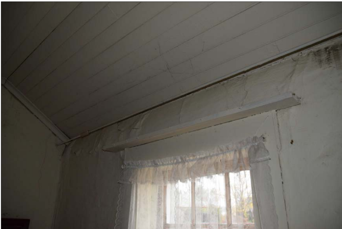
Figure 23: The head of the front wall with cracking and signs of water ingress. Photograph: Origin Consultants
