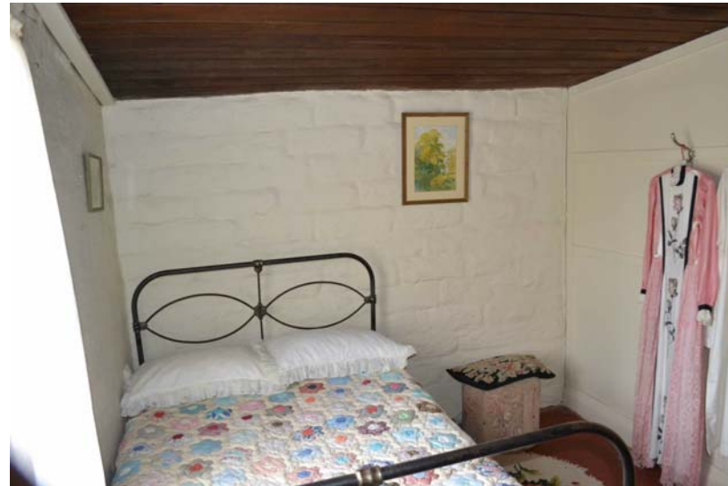
2. Room 3 with unplastered painted mudbrick wall at the rear of the room, there is significant decay at the base of the wall.
