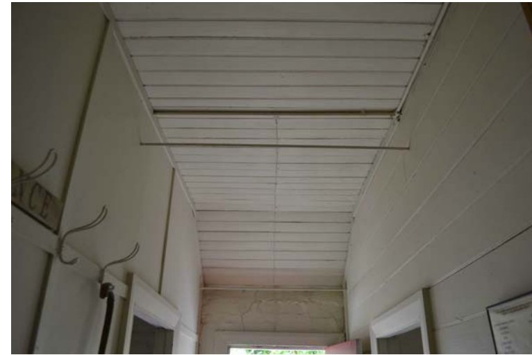
3. Room 5 showing steel tie at high level.
