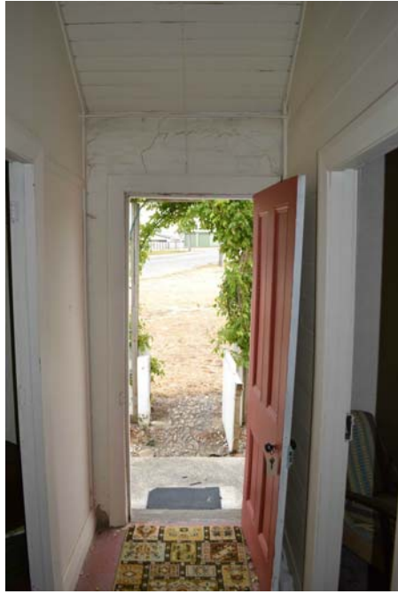
1. Room 5 front door with no threshold and cracks above the door.
