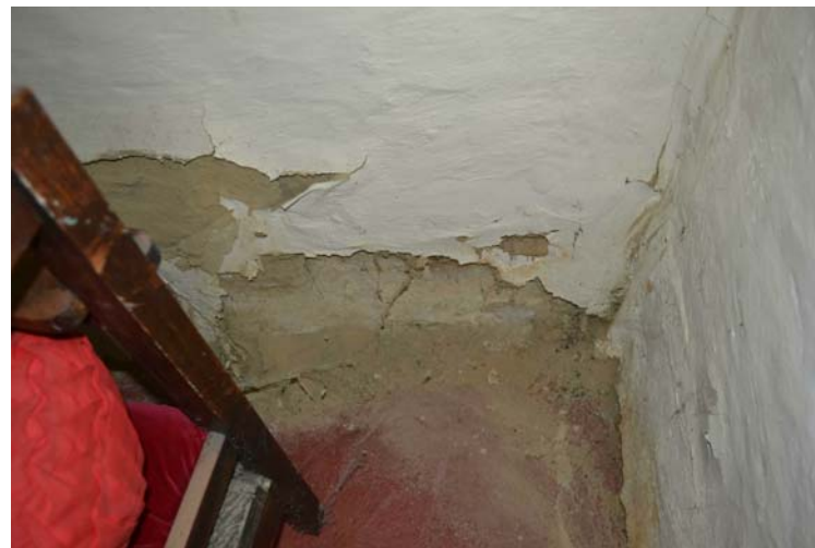
4. Room 3 decay in the base of the earth wall with plaster broken off and wall disintegrating.
