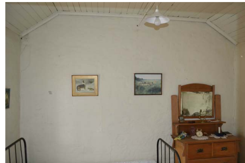
3. Room 1 showing the T&G ceiling and rods at high level. There is cracking in the walls at both corner junctions.
