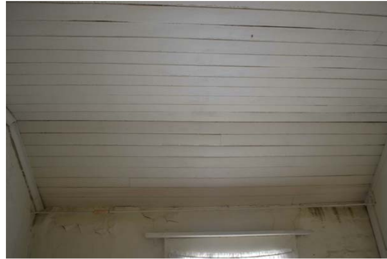
2. Room 1 Water damage and movement of wall at eave level and sagging to some T&G ceiling boards.
