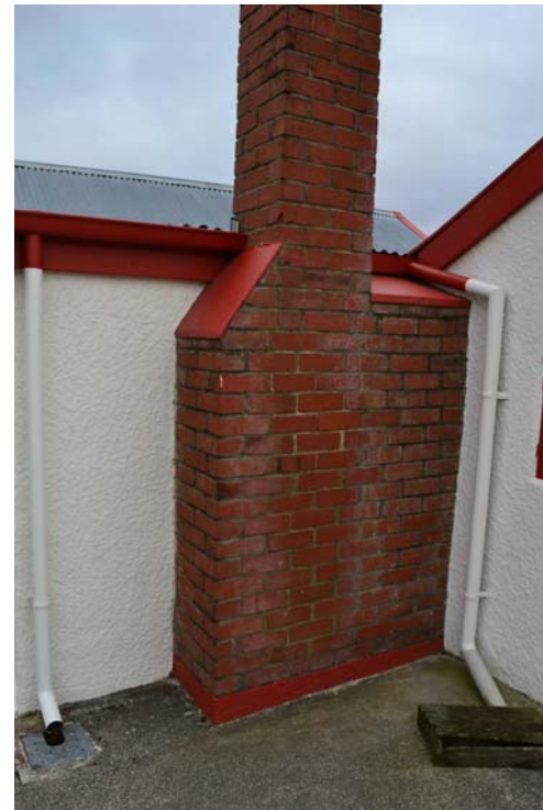
6. Late 20th Century brick chimney at rear of building cast on a concrete pad with the scullery to the right.
