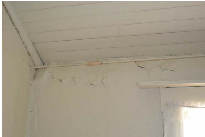
1. Room 1 water damage and movement in the wall head at eave level.
