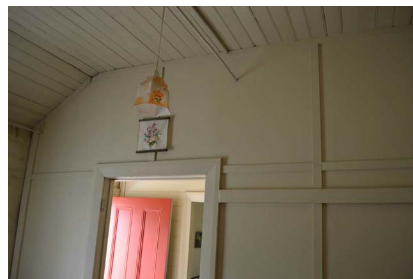
5. Room 2 timber framed internal wall with lining and panelling. Tie rods at high level.
