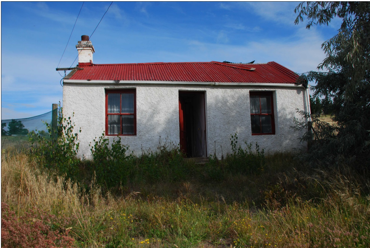
Figure 19: The earth cottage at Peyton's Patch, close to Vallance Cottage, which was demolished in 2012. Photograph: Origin Consultants
