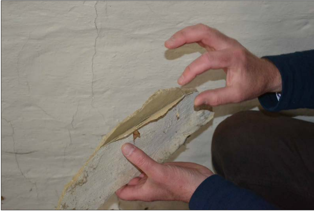
Figure 18: A detached section of painted, earth plaster skim to one of the internal walls. Photograph: Origin Consultants
