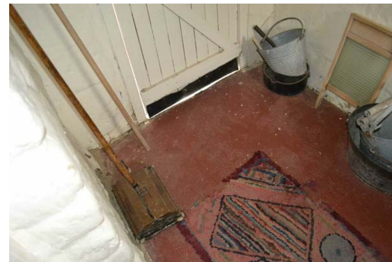
6. Room 6 showing the concrete floor and gaps under at the exterior door.
