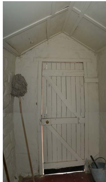
5. Room 6 with cross braced panel door. Note the different wall to the right of the photo.
