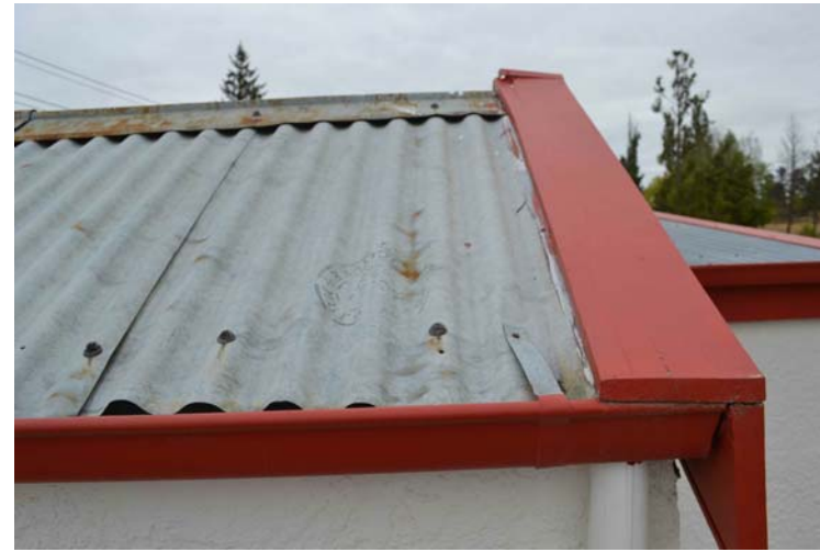
5. Roofing over Room 6 with raised nail heads.
