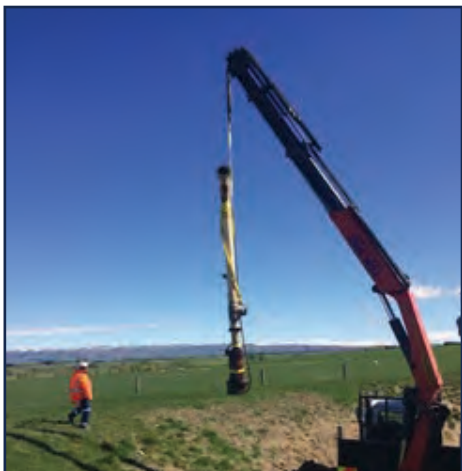
The Backwash pump removed from the reservoir
