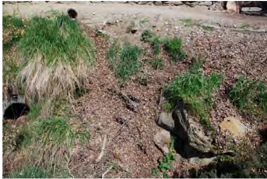
Water flows between the anchorages, which are likely to be clogged by debris. Remaining cables are likely to corrode more quickly.
