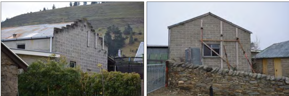
Figure 29: The Briar Herb Factory building (F) east elevation (left) and west elevation (right) with modern propping in place.
