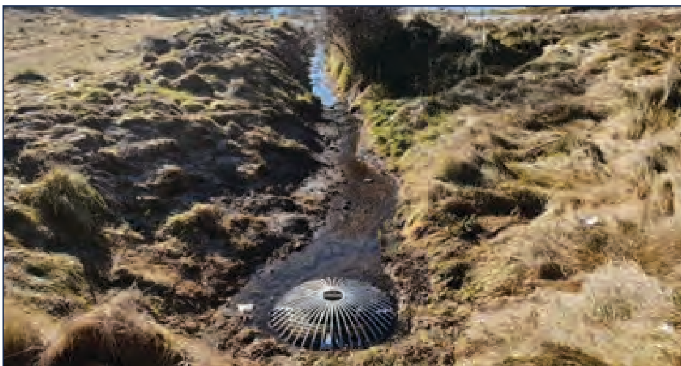
Scruffy dome on stormwater inlet
