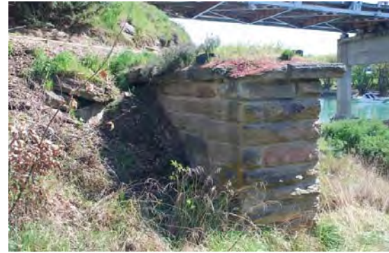
The bank is spreading and building up behind the small south pier/abutment.
