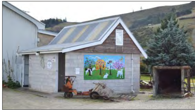
Figure 28: The concrete block public toilets located to the east of the Goods Shed and Blacksmiths.
