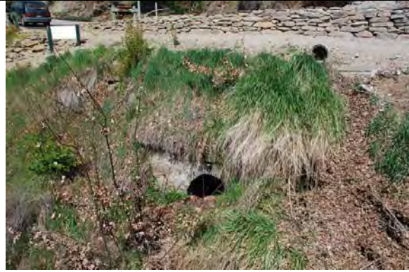
Surface water outlet directly above one of the anchorages – leaves indicate the main flow of water from the outlet
