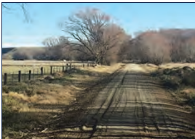
Freeze thaw conditions – Auripo Road – August 2018
