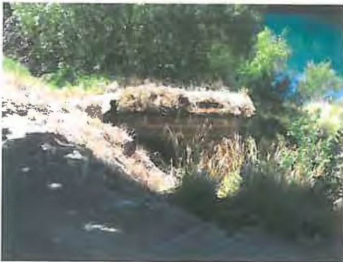
View of intermediate support pier between old abutment and main pier on Roxburgh side of river. It may be possible to restore this pier including the replacement of the original masonry pillars on each side
