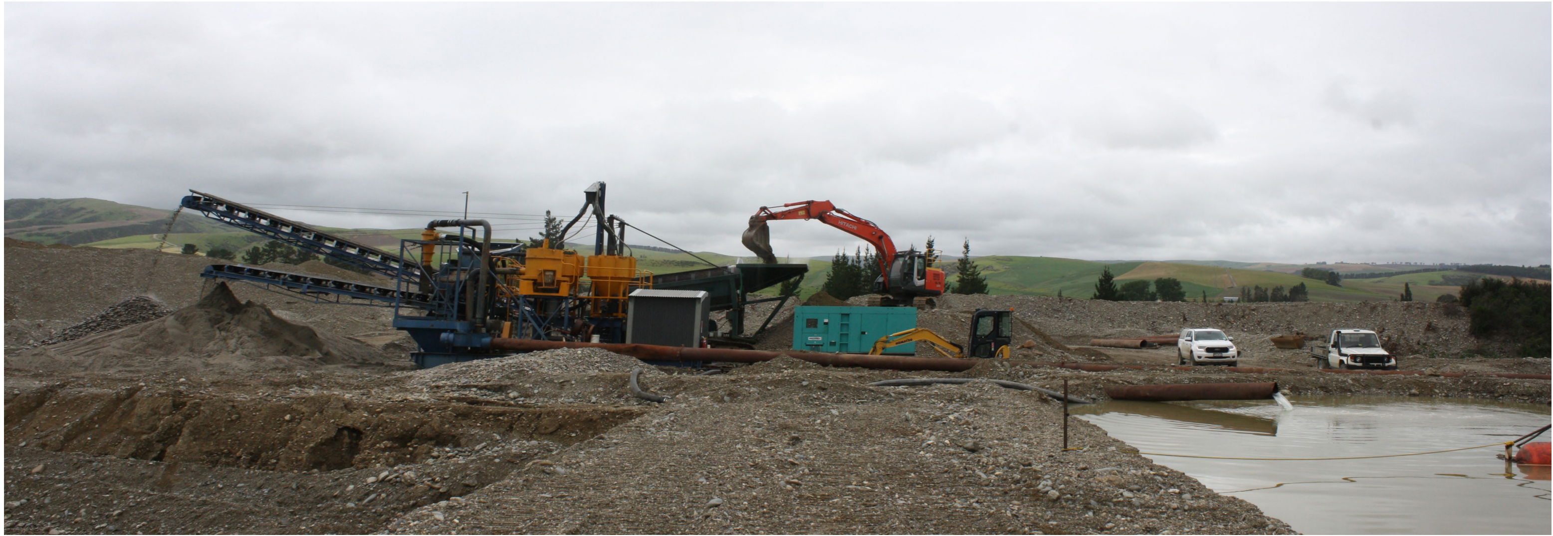
Figure 13: The processing plant already present on the site for the exploratory works.
