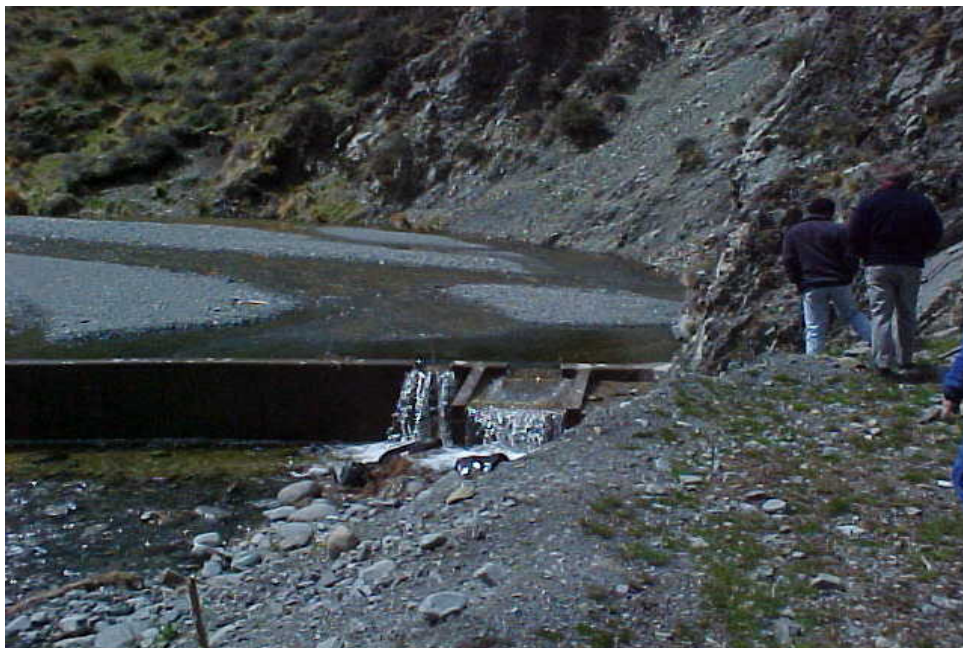
Ranfurly intake weir
