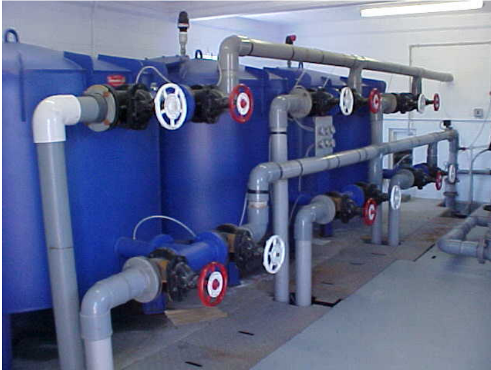
Pressure Sand Filters
