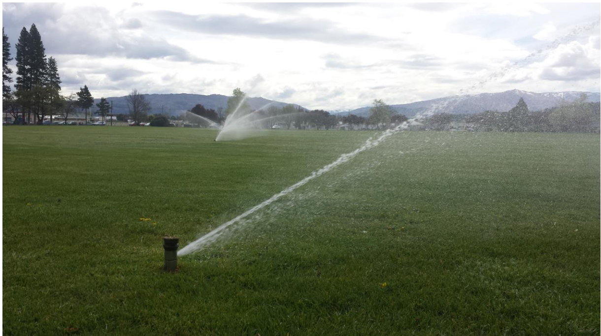
Pop-up irrigation operating within the park
