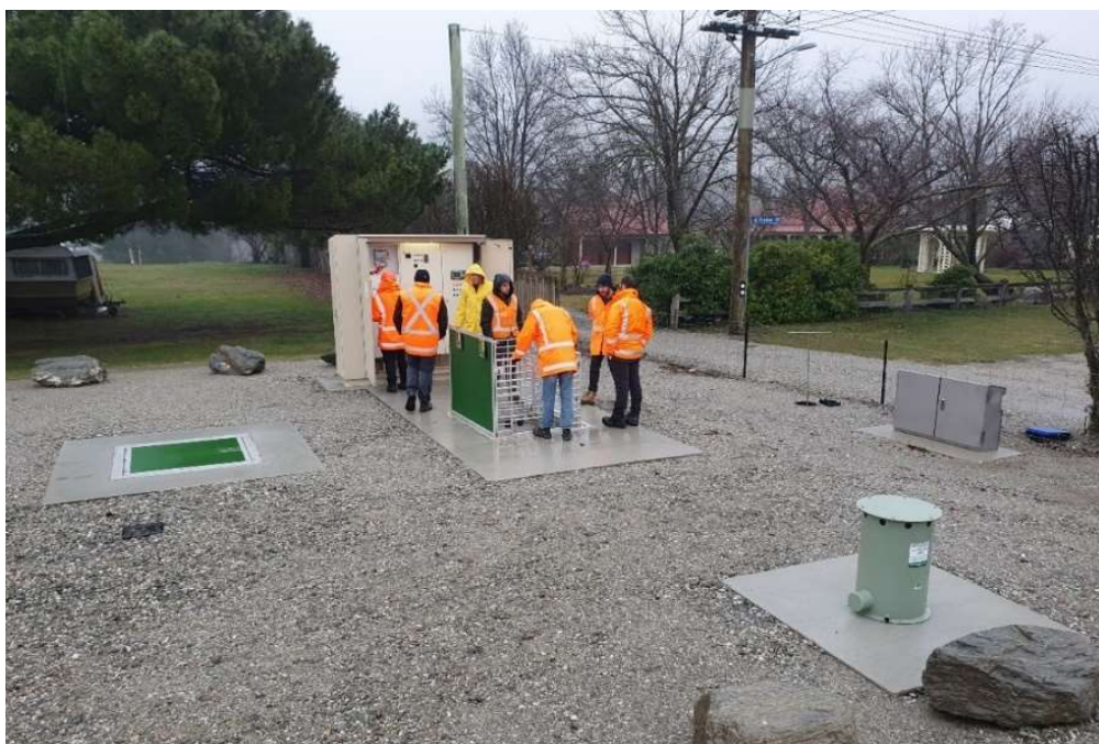
Figure 7: Pump station at Clyde Camping ground
