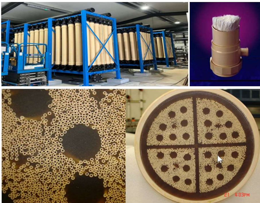
Figure 2: The three membrane racks at the water treatment plant
