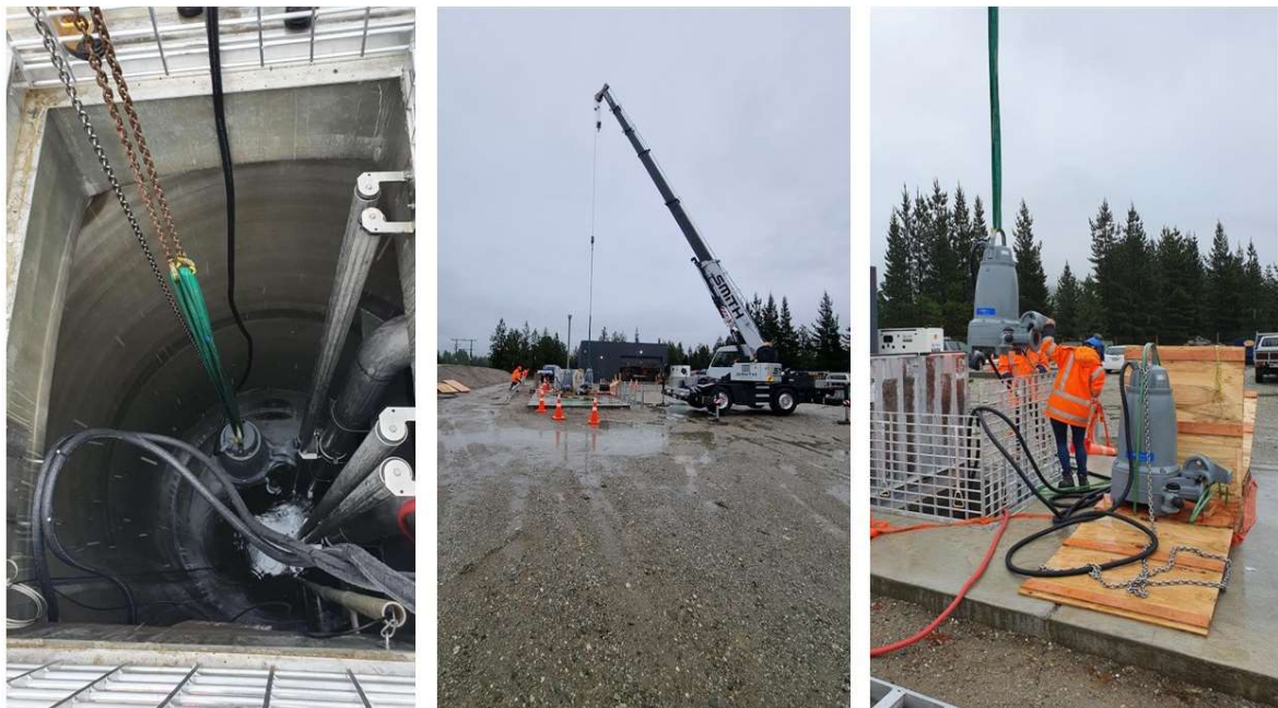
Figure 8: Commissioning of the Clyde main wastewater pump station. Pumps being installed into the 6m deep wells
