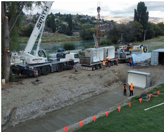
Figure 9: Drone photo of storage installation
