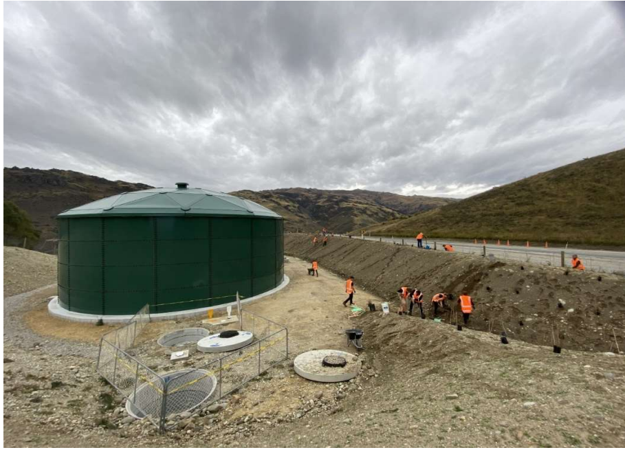
Figure 1: Lake Dunstan Water Supply
