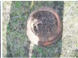
Full pipe blockage
