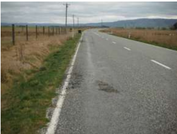
Seal failure on Ida Valley Road
