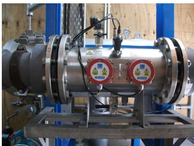
UV treatment Roxburgh Water treatment plant
