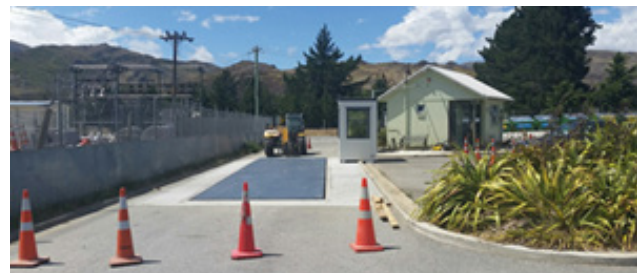
Cromwell Transfer Station Weighbridge
