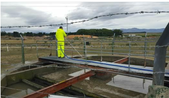
Fulton Hogan Operator carrying regular maintenance on the Ranfurlly Waste Water Treatment Plant
