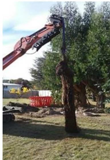
A major root blockage was discovered in Roxburgh and was cleared out from the main storm water pipe.
