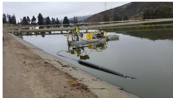
A dredger is used to collect sludge from the bottom of the Oxidation ponds.
