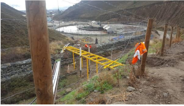
Earlier picture of the tanks foundations. The pipe bridge (foreground) is painted yellow so that mountain bikers can pass it safely.
