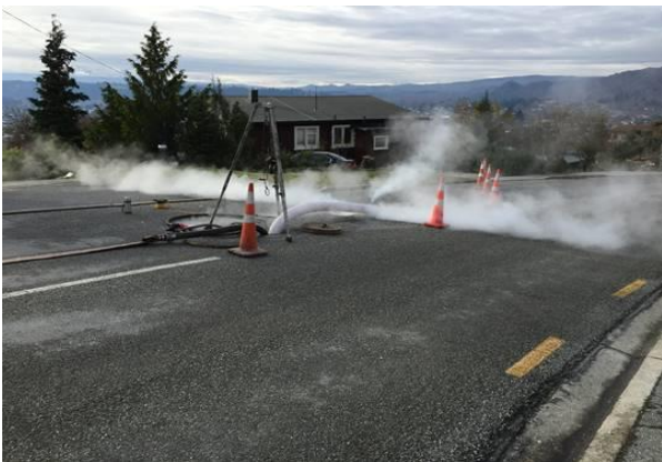
The new pipe liner involved rehabilitation of a 160m long section of earthenware sewer.
