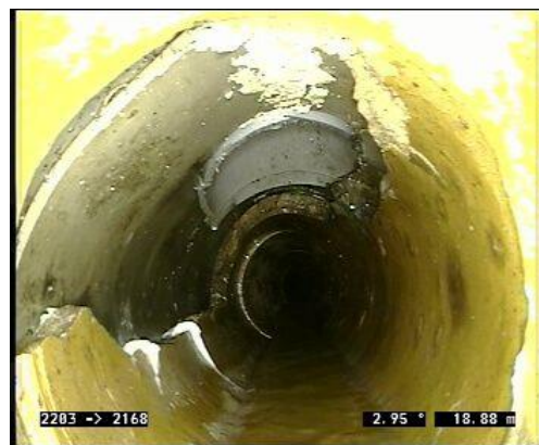
One of the sewer pipes in Naseby with fallen concrete.
