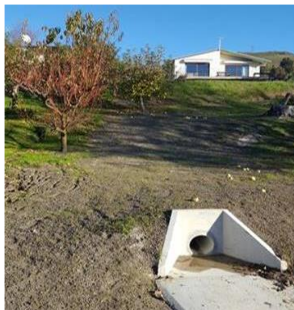
The pipe allows storm water to flow away from areas previously prone to surface flooding within properties
