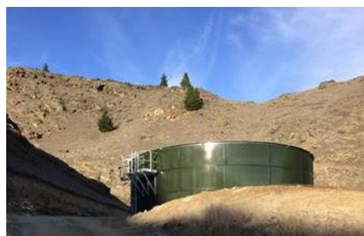
Partially completed balance tank for the new UV Plant. The pipe bridge is painted yellow so that mountain bikers can pass it safely.
