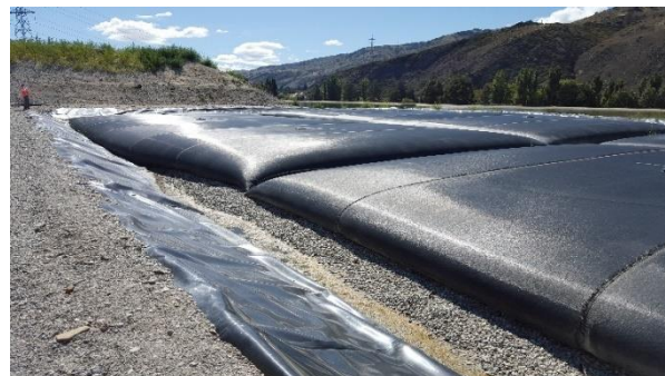
'Geobags' are used to store and dry the collected sludge. The Geobags will eventually be covered with soil.
