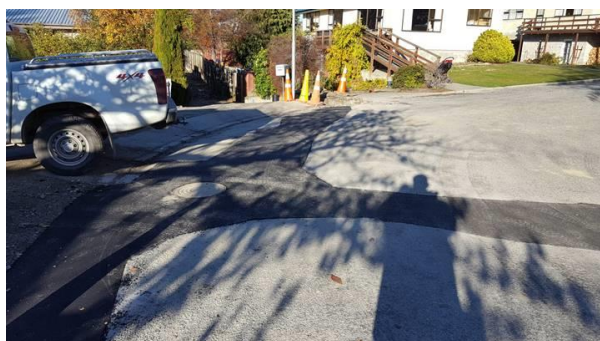
Storm water pipe is now reticulated off the road surface and into the newly installed pipe.
