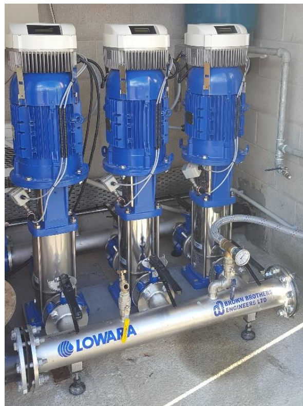
New Booster Pump System with improved pressure control and capacity.
