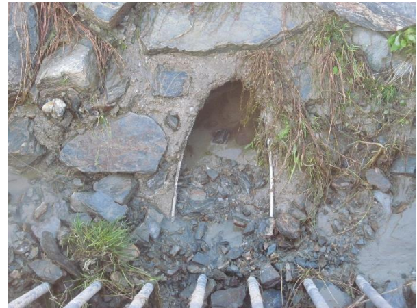
Inspection of stormwater pipe in Roxburgh, which was found to be partially blocked and required clearing.
