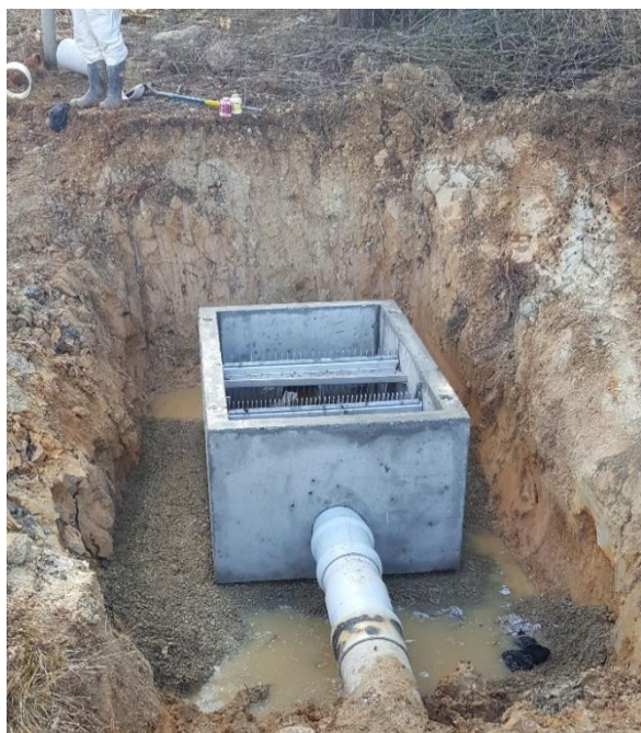
Naseby WWTP Screen
