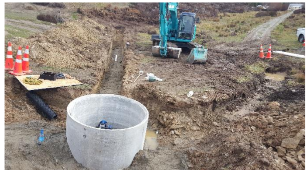
New pressure valve chamber.
