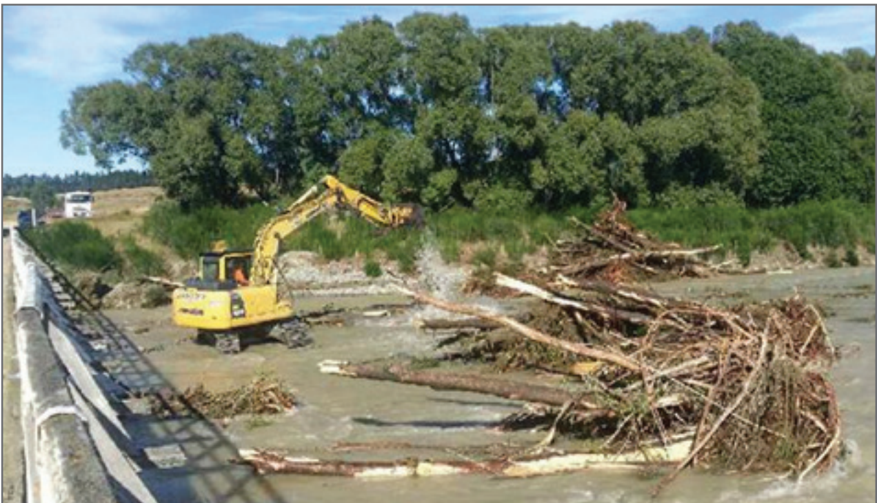
January - Fulton Hogan clearing log jam from underside of Scotts Lane Bridge
