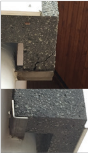
Cracks were identified at both ends of the concrete support frame where the bolts are inserted.
