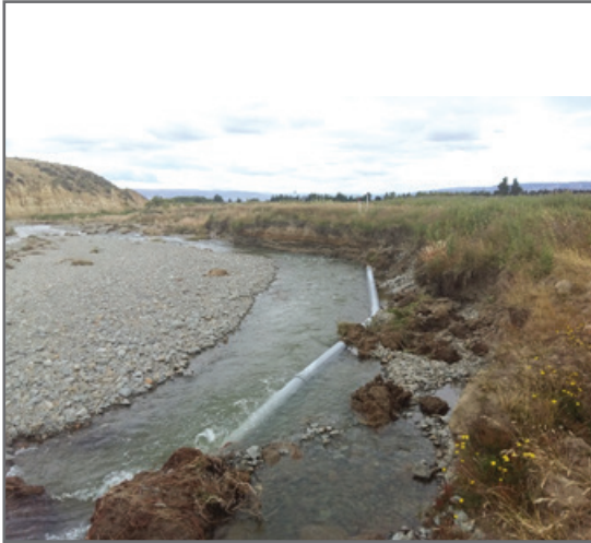
Changes to river flow path caused erosion of the bank
