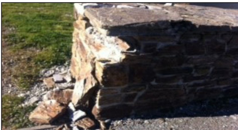
Damage to the stone wall at the Junction was identified and work will be undertaken to fix this.
