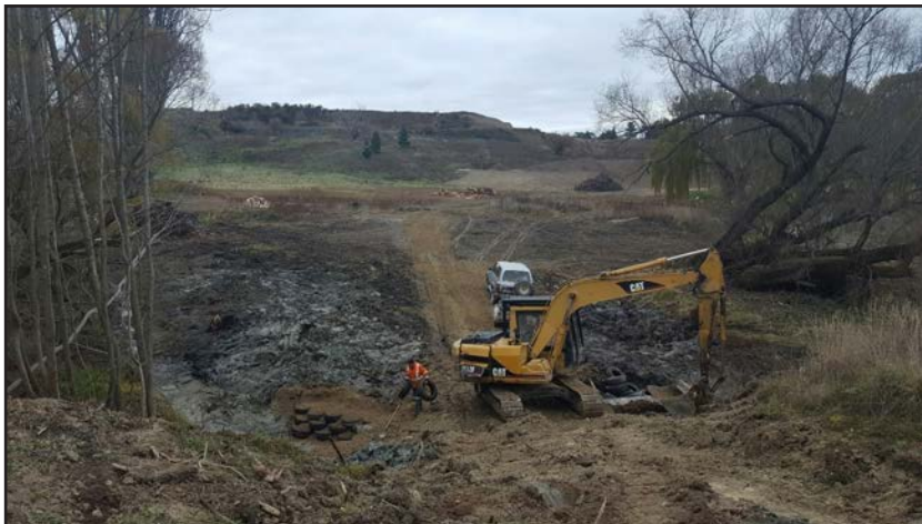
Work progressed on the development of the Bannockburn Track, at the Schoolhouse Road end.
