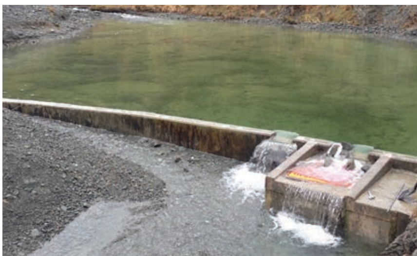
Nicely cleaned out intake weir for Ranfurly water supply
