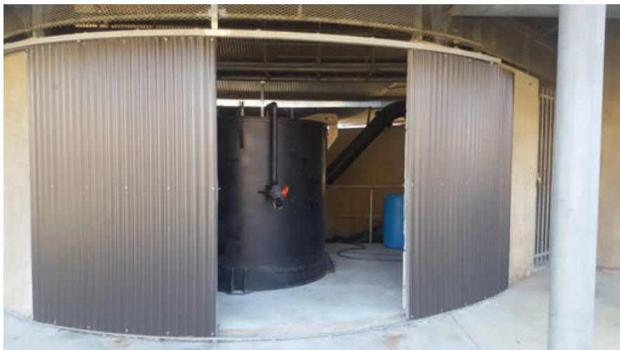
New door and chlorine tank
