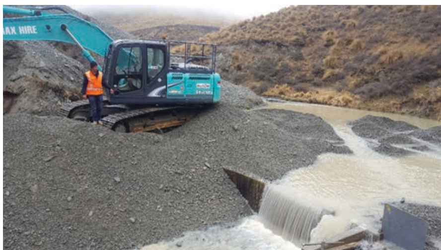
Ranfurly intake weir full of river gravel during extraction
