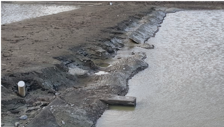
Damage at Omakau Wastewater Plant
