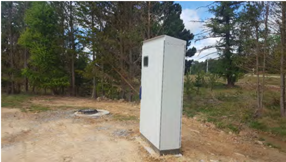
Flow meter chamber and electrical control box.
