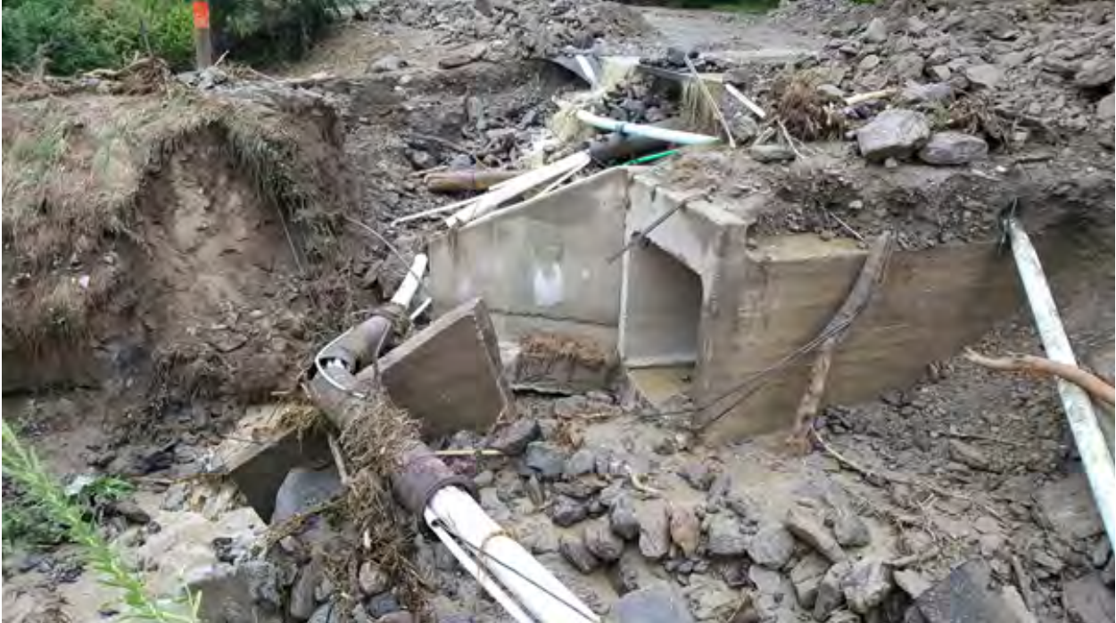
Roxburgh Pump Station Creek culvert after the rain event.
