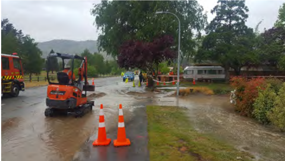
Flooding created by damaged main.
