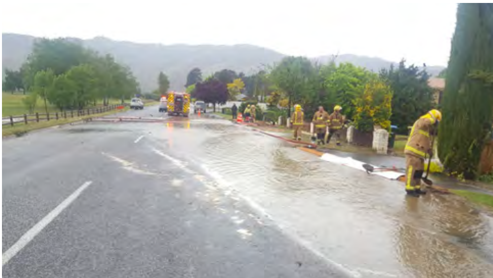
Flooding from damaged main, with assistance from the Fire Service.
