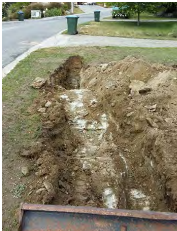
Large rock in the trench on Aronui Road, Alexandra.
