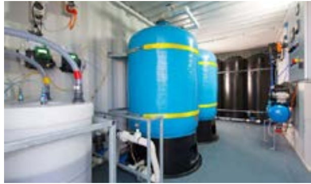
Inside the portable water treatment plant.
