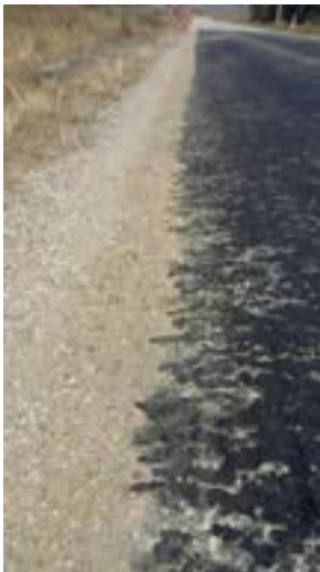
Bleeding seal on Ranfurly Patearoa Road
