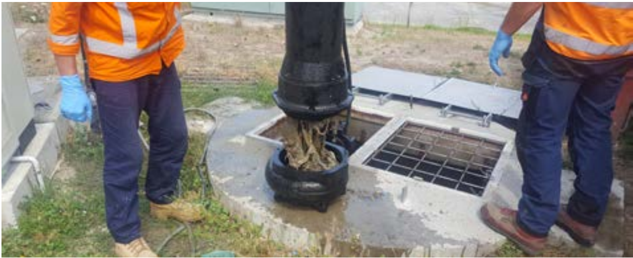
Fat, rags and wipes blocking a pump.
