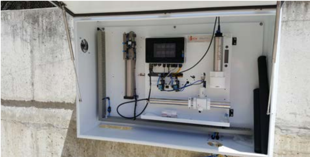
S::CAN Wastewater Monitoring Equipment.
