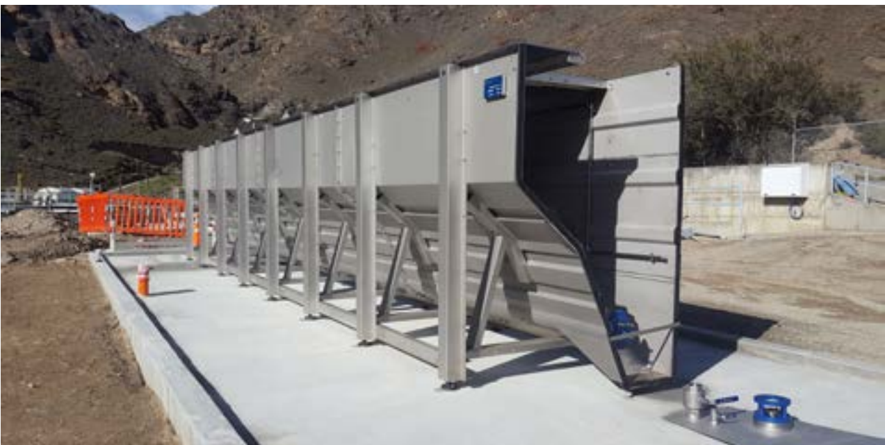
New screen in place at the Alexandra plant awaiting assembly and connection.
