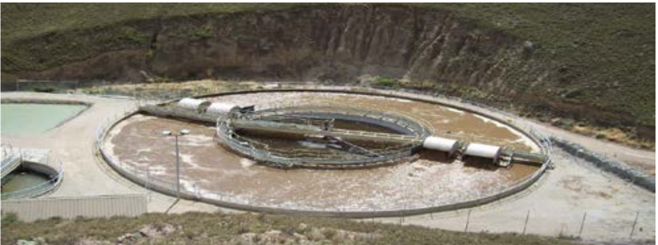
Aeration ditch with four aerators
