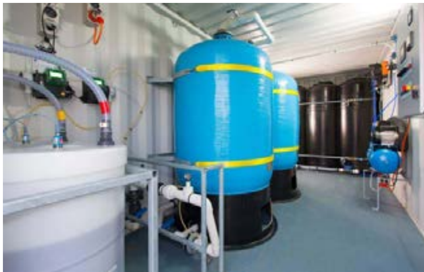
Inside the portable water treatment plant
