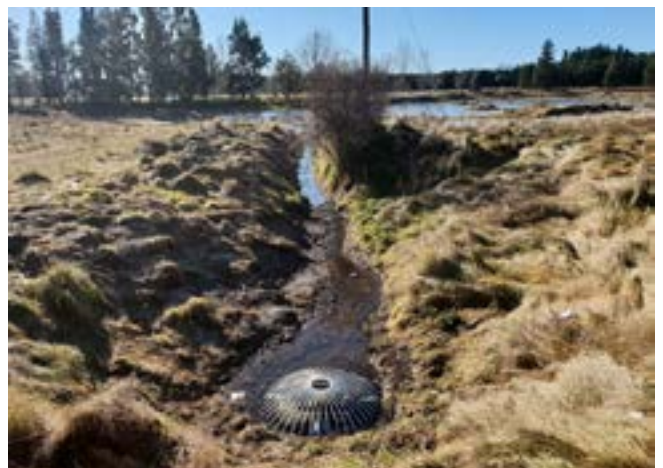
Scruffy dome on stormwater inlet
