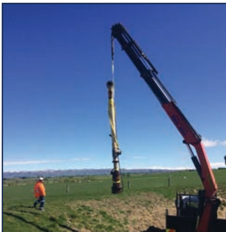
The Backwash pump removed from the reservoir
