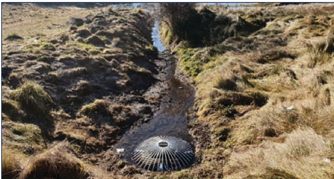
Scruffy dome on stormwater inlet
