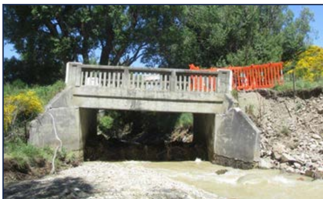
Bridge 94 slumping badly on the right. Flood waters gouged bank behind and under the right wing wall and abutment
