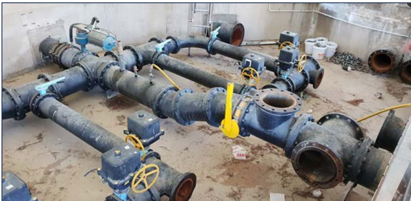
Old pipe work at the Cromwell Water Treatment Plant.
