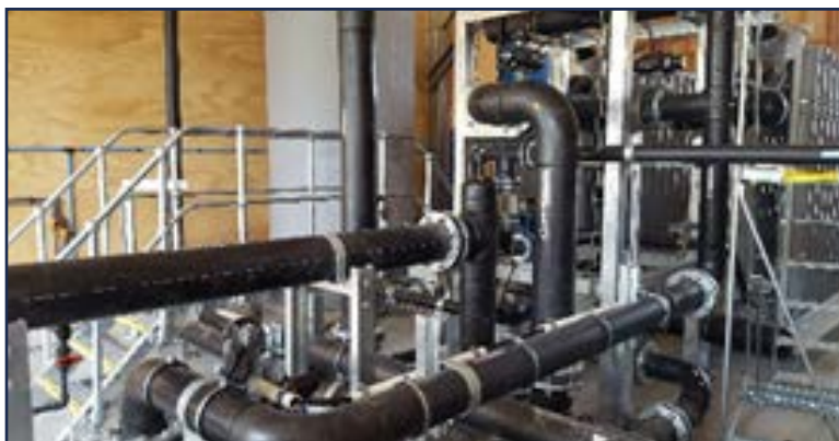
The internal filters at the waste water treatment plant.
