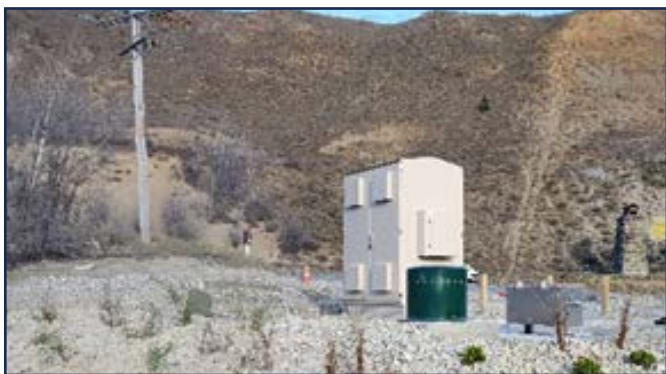
Bannockburn pump station which transfers wastewater to the Cromwell treatment ponds. Wastewater is no longer discharged from the Bannockburn area to the Kawarau Arm of Lake Dunstan.
