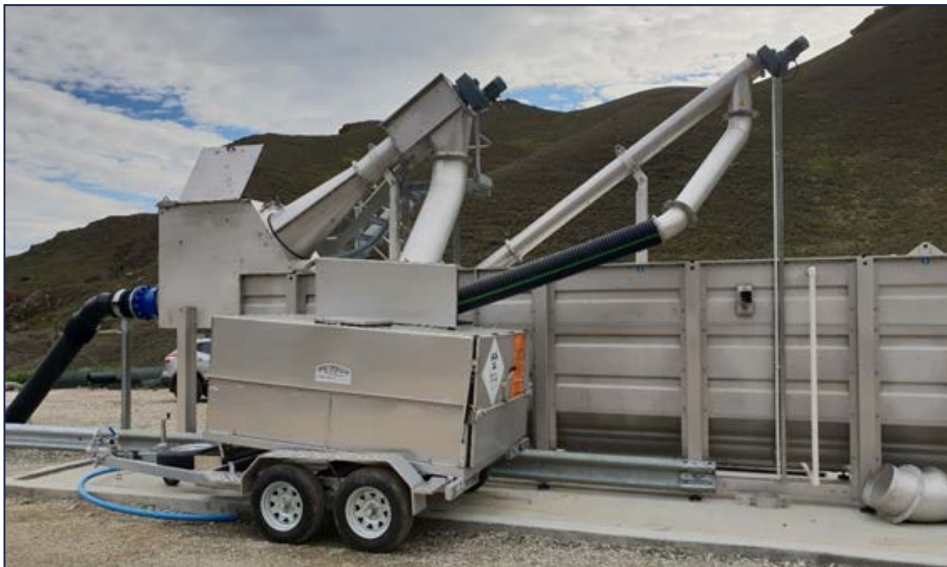
New inlet works and screenings trailer.
