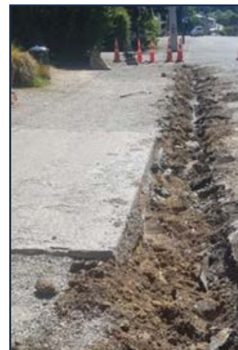
Kerb replacement on Derwent Street. Old kerb being removed ready for new kerb pour.
