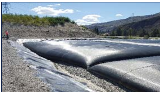
Sludge bags before covering. Removal of the sludge was the first step in the upgrade of the Cromwell wastewater ponds.
