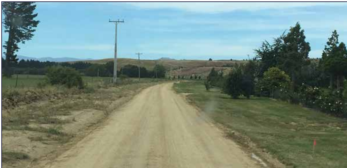
Booth Road. Road was shaped and water channels installed to improve drainage and extend lifespan prior to eco sealing – January 2019
