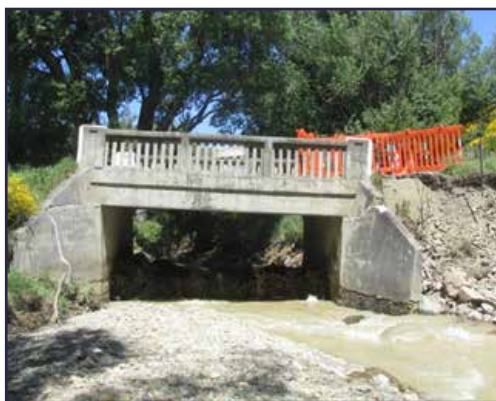
Bridge 94 slumping badly on the right. Flood waters gouged bank behind and under the right wing wall and abutment
