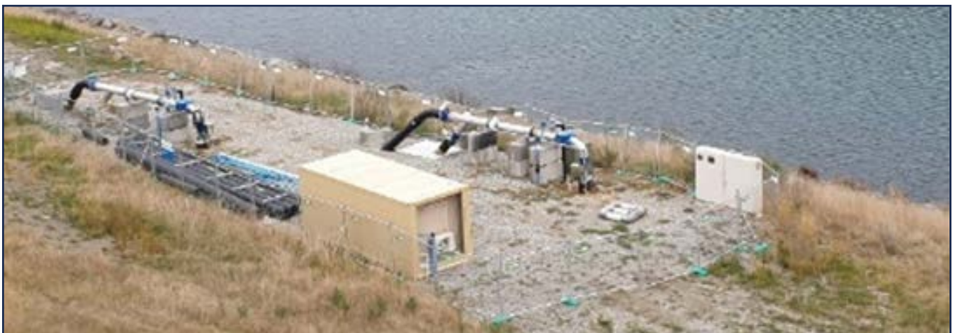
Bore field where water is drawn from approximately 25m underground beside Lake Dunstan near Clyde.
