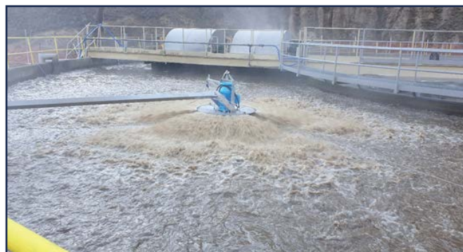
First aerator in the aeration ditch and operating.
