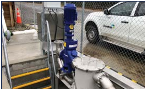
The blue muffin monster can be seen next to the rock trap.
