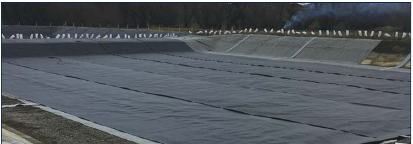
Installation of the liner to pond one at Omakau Wastewater Treatment Plant
