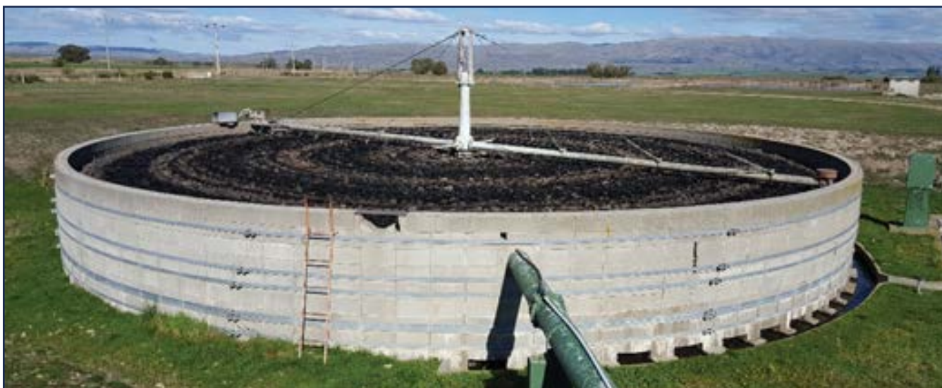
Ranfurly wastewater treatment plant trickle filter.
