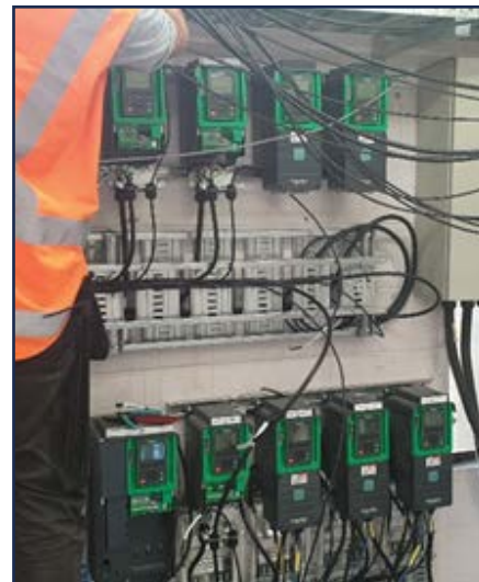
Motor Control Centre showing the VSD's mounted on the wall.
