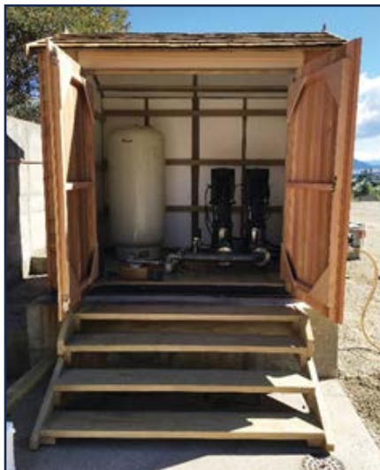
Relocated service water pumps in new shed.
