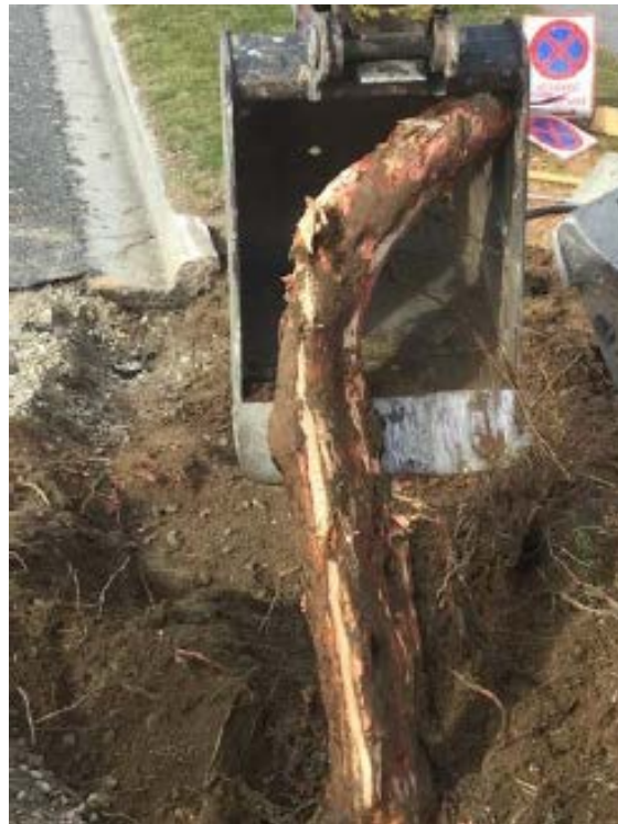
Tree root removed from kerb and channel - Gair Ave
