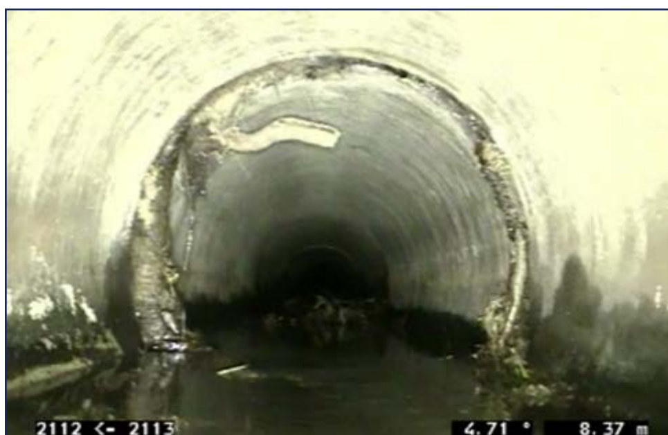
CCTV image of the root intrusion.
