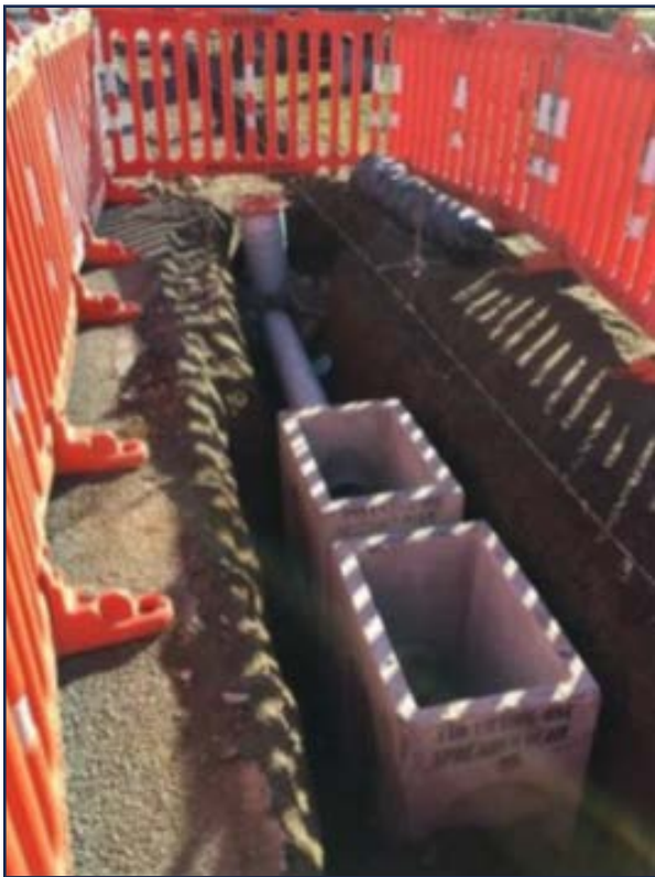
Mudtanks connected to soak pits, McNulty Road – July 2019
