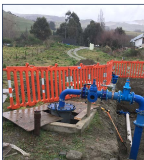
Improved bore headworks and connecting pipes.
