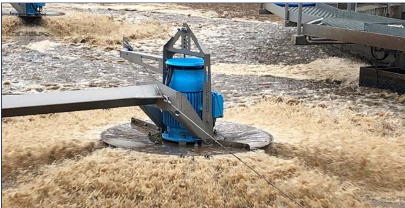
Aerator in action.
