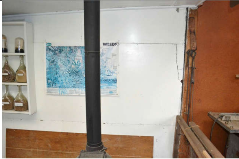
Building G – some internal linings may contain asbestos fibres
