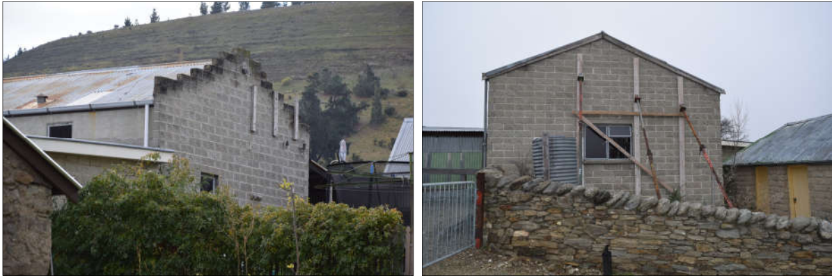
Figure 11: The Briar Herb Factory building (F) east elevation (left) and west elevation (right) with modern propping in place.
