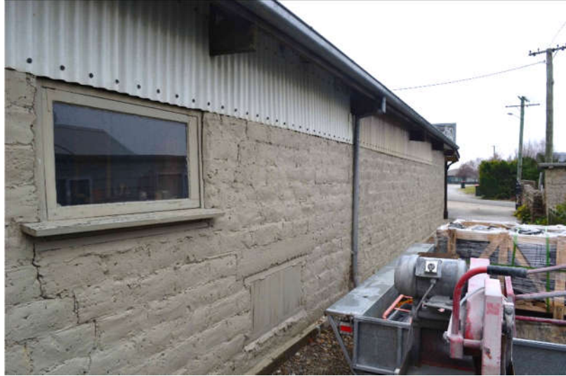
Part of the mud brick south wall with timber and fiberglass upper wall.
