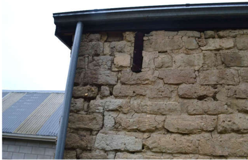
Cracking and loss of mortar in mud brick wall
