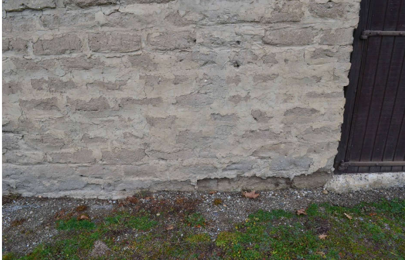
Poor repointing and mud brick decay near foundation
